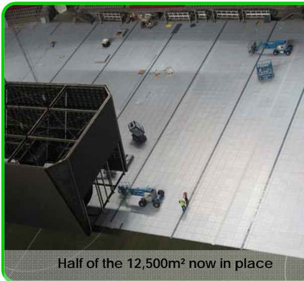
Moveable seats rolling out on top of terracover“V” ®
